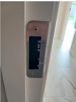
Photo 12 Kitchen/hall door — strike/keep alignment detail. 20260903_083140.jpg
