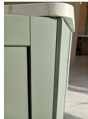
Photo 18A Kitchen island — outer cabinet door contacting gable/end panel. 20260903_084138.jpg
