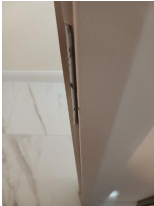
Photo 21B Under-stairs store — strike/architrave alignment detail. 20260903_084300.jpg
