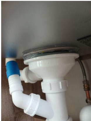
Photo 20 Utility sink — waste outlet/seal junction where moisture was detected. 20260903_084227.jpg
