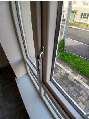
Photo 14 Front living room — smaller window operation/closure issue. 20260903_083324.jpg
