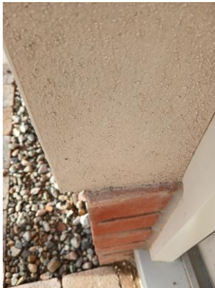
Photo 23 Utility door exterior — incomplete render corner/junction. 20260903_084625.jpg
