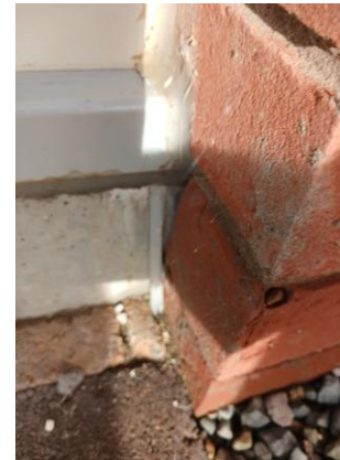
Photo 24 Utility door exterior — inconsistent brick/render junction. 20260903_084525.jpg
