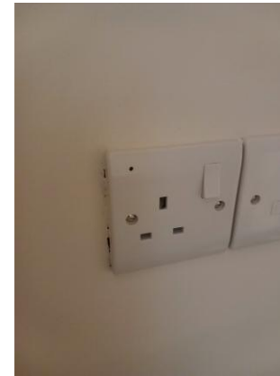
Photo 05 Drying cupboard — local unfinished gap beside socket faceplate. 20260903_082536.jpg
