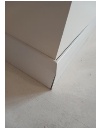
Photo 03 Upper floor — skirting section cut but not fixed. 20260903_082212.jpg
