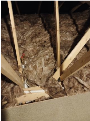
Photo 01A Roof space — disturbed and uneven quilt insulation coverage. 20260903_081917.jpg
