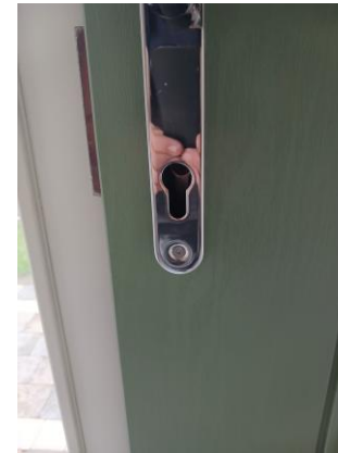
Photo 07 Entrance hall — permanent front-door cylinder arrangement incomplete. 20260903_082709.jpg
