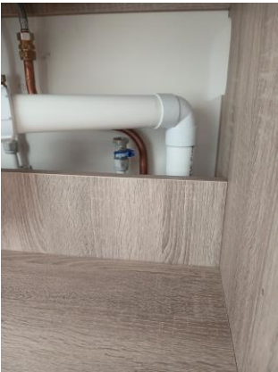
Photo 29 Utility room — washing-machine service points below sink. 20260903_084458.jpg
