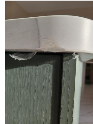
Photo 19 Kitchen island — damaged/scratched worktop finish near corner. 20260903_084110.jpg
