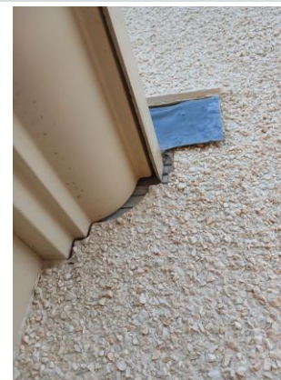
Photo 09A Front canopy — incomplete rendered junction at one side. 20260903_082817.jpg
