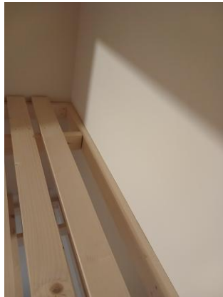
Photo 06 Drying cupboard — incomplete rear shelf support/infill. 20260903_082604.jpg
