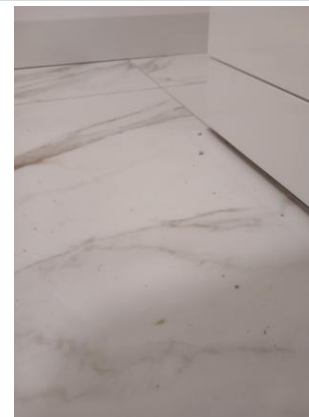
Photo 10 Ground floor — construction debris remaining on finished floor. 20260903_082939.jpg
