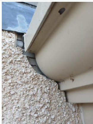
Photo 09B Front canopy — incomplete rendered junction at opposite side. 20260903_082824.jpg
