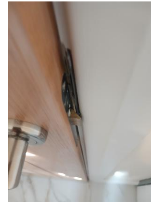
Photo 21A Under-stairs store — latch obstructed by tight architrave margin. 20260903_084258.jpg
