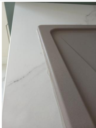
Photo 17 Kitchen — excess sealant at sink-to-worktop perimeter. 20260903_083738.jpg
