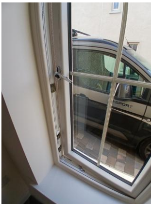
Photo 13 Front living room — main opening window did not lock securely. 20260903_083204.jpg
