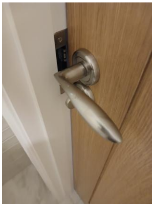
Photo 11 Ground-floor bathroom — door-latch engagement issue. 20260903_083122.jpg
