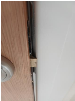
Photo 02 Rear right bedroom — latch contacting tight architrave margin. 20260903_082200.jpg
