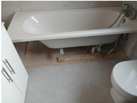
Photo 04 Main bathroom — bath side closure/panel absent. 20260903_082234.jpg
