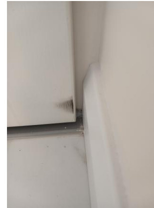
Photo 22 Utility external door — black mark at lower right-hand corner. 20260903_084410.jpg
