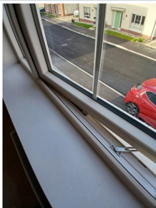
Photo 15 Front left bedroom — opening window caught during operation. 20260903_083402.jpg
