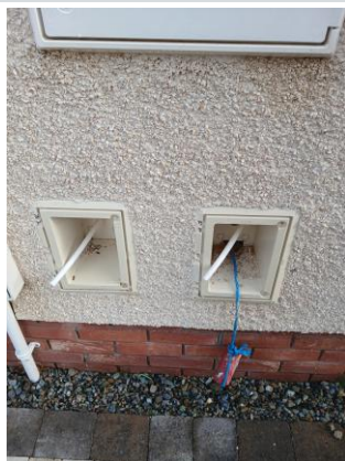
Photo 08 Front exterior — two service boxes without external covers. 20260903_082739.jpg
