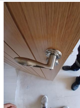
Photo 16 Main bedroom en-suite — loose door handle. 20260903_083500.jpg
