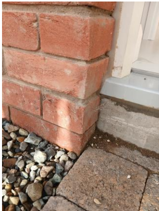
Photo 25 Utility door exterior — projecting brick and uneven mortar margins. 20260903_084634.jpg
