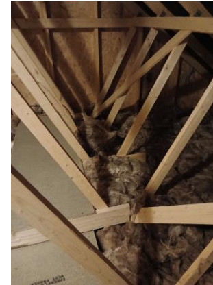
Photo 01B Roof space — detail of quilt insulation displaced around services. 20260903_081931.jpg
